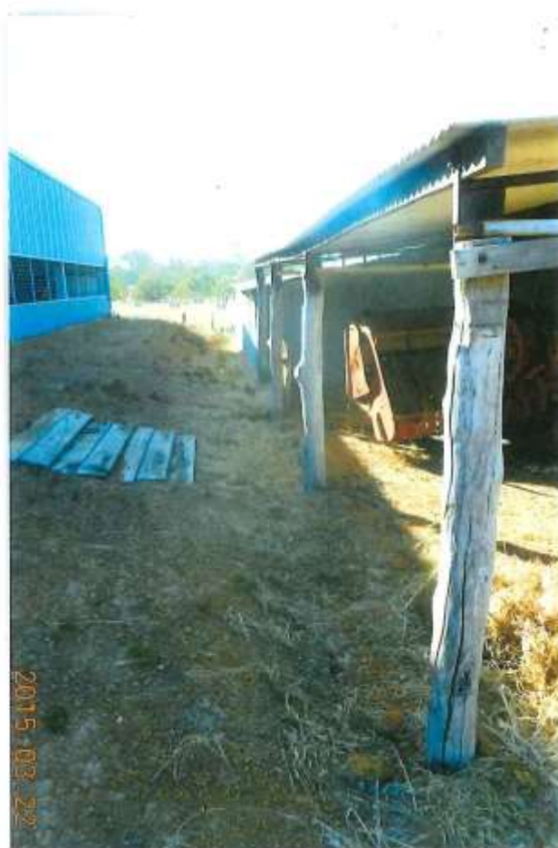
PROPOSED WALL WILL GO FULL LENGTH OF SHED WALL 900mm HIGH TO HOLD BACK GRAVEL TO FILL SPACE UP TO SHED
